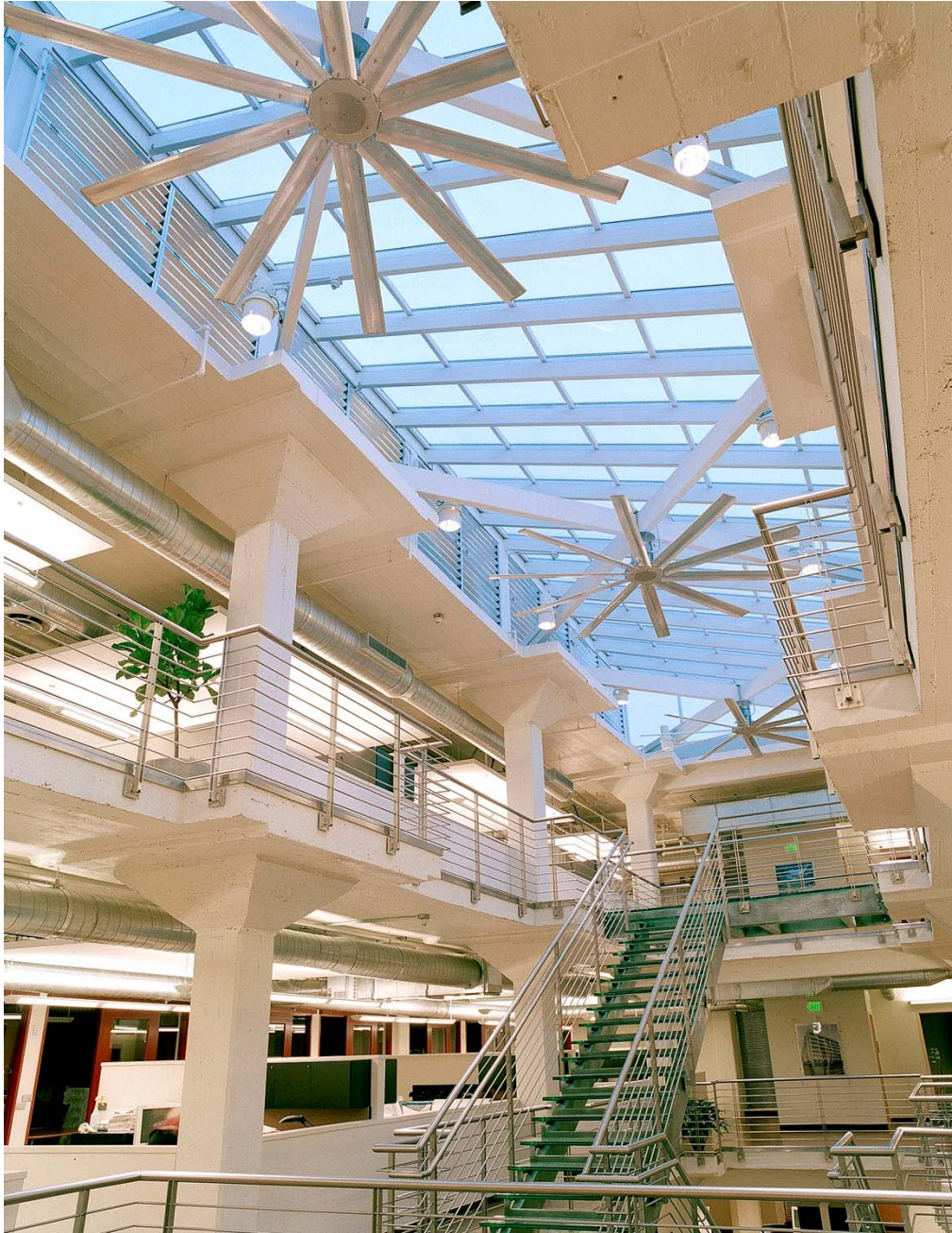
Figure 10. An atria fitted with HVLS circulating fans for de-stratification.
