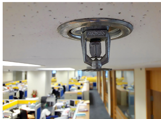
Automatic ceiling fire sprinkler installed in an office.
