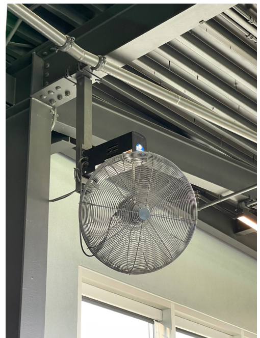
FIGURE 4. Air-circulating fan head mounted to a ceiling beam.
