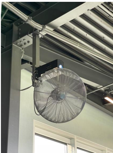
Figure X: Photo of an air circulating fan head mounted to a ceiling beam. The fan cannot be tested to AMCA 230, but may need to meet the design requirements of a ceiling fan. Photo courtesy of AMCA International.
