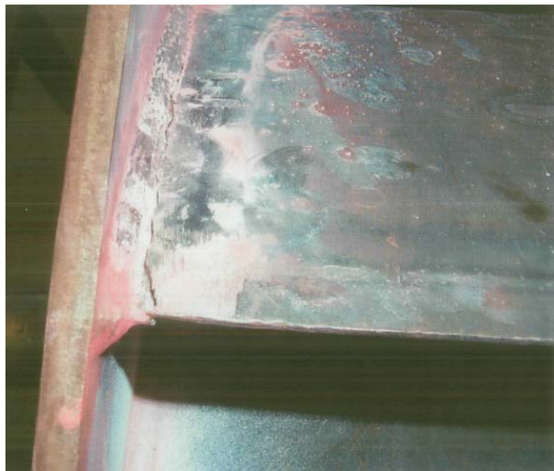
Figure 24. Impeller, Experimental Fatigue Test, Blade Crack Detail #1
