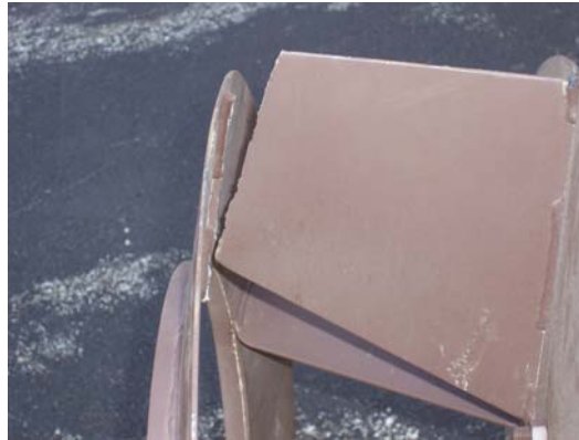
Figure 19. Cracked Impeller Blade
