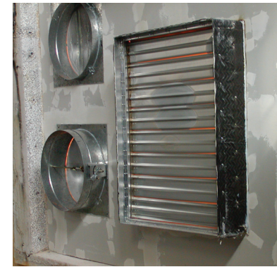
Figure 5b: An “out of the wall/partition” fire damper installed on a 2-hour-rated steel/gypsum firewall. Photo courtesy of United Enertech.
